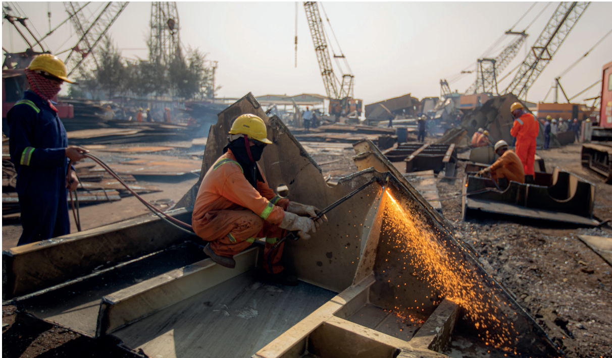
Werkers op scheepsloopwerf. Leela Greenship recycling PVT PLT PLOT no. 35, Panchvati ship breakers plot no.20, Alang, Gujarat, India
